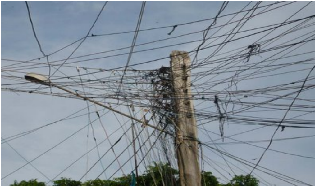
Figure 11 Example of an illegal electric energy connection in a favela of the Municipality of Rio de Janeiro Source: O Globo, 2011.
